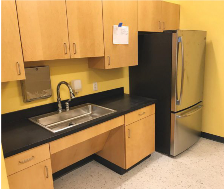
Residential appliance and washroom accessories were installed in the kitchen of the State of Connecticut Department of Transportation building in Waterbury, Connecticut.
