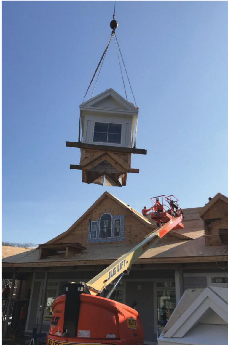
Elite Construction Rentals LLC installs the cupola at Maplewood at Southport, a senior living community in Southport, Connecticut.
